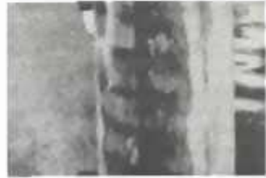
Corroded reinforcing steel in a concrete column exposed to salt water. Corrosion of the steel has caused severe spalling of the concrete.
